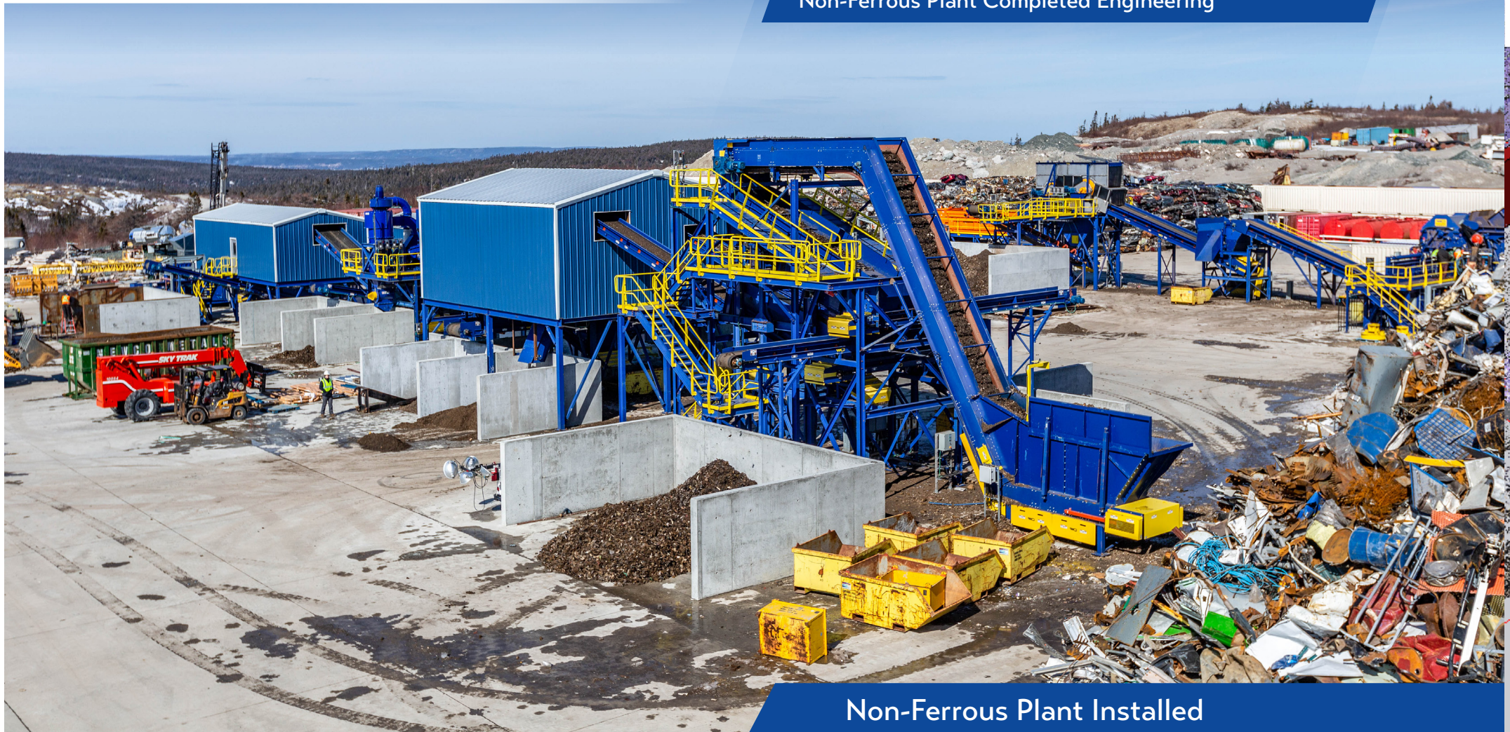
Non-Ferrous Plant Completed Engineering
